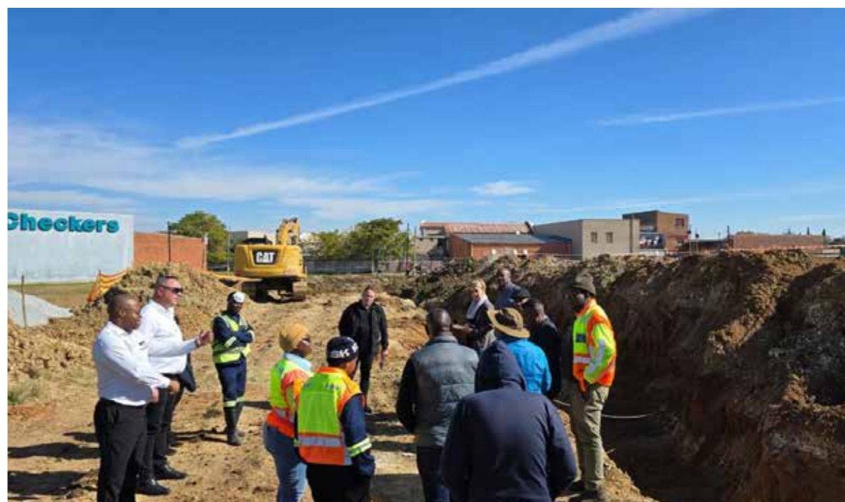
Representatives from DWS, Matjhabeng LM and Checkers doing a site visit on the work currently underway to eradicate sewage spills in the area of St Helena in Welkom. Picture: Supplied
