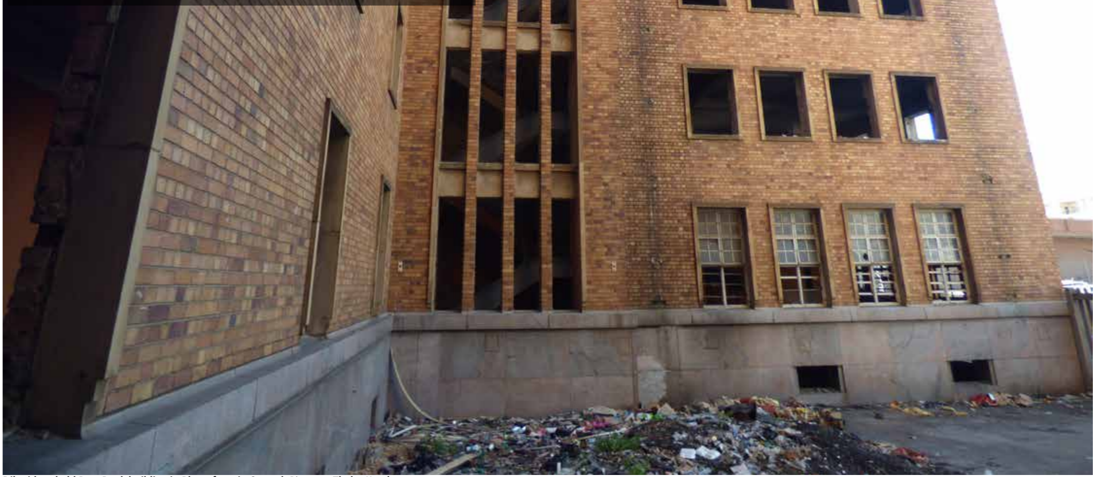
Dilapidated old Post Bank building in Bloemfontein Central. Pictures: Thabo Ketele
