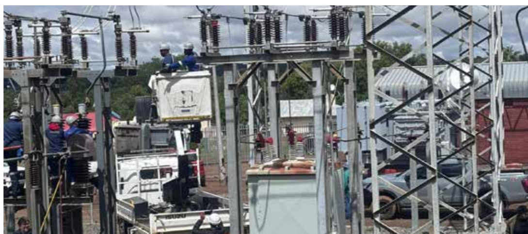
Centlec technicians worked around the clock to restore power following the transformer blast. Picture: Facebook
