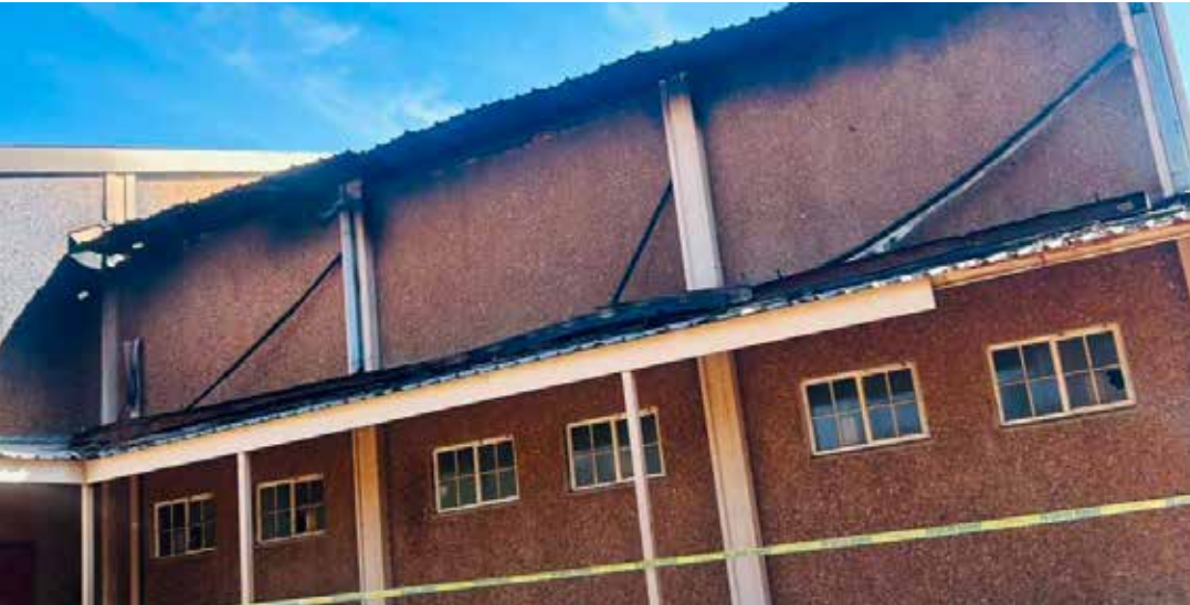
Two school fires in the North West province within three days have damaged critical infrastructure, putting further pressure on already limited resources. Picture: Supplied
